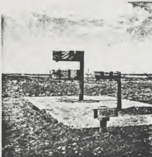
FIGURE 15. SITE AG 205 ROUND I. TYPICAL INSTALATION
